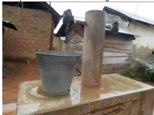
Figure 4.6 Cracked and eroded concrete platform, defective taps and a girl fetching water at Mampong
