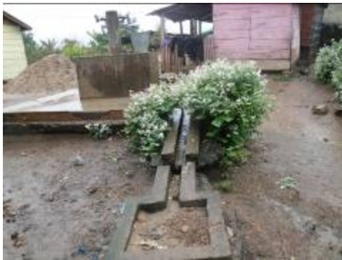
A cracked drain and eroded platform
